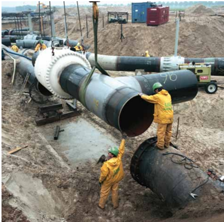
A.Hak did a great job in a 1986 project near Ommen, where a compressor station was modified and expanded for Gasunie.
