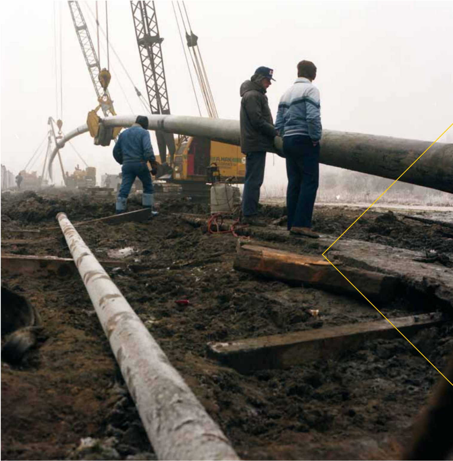
The first horizontally directed drilling in Western Europe is completed by A.Hak in cooperation with the Texan firm Berco. Here, the Buiten-IJ lake is crossed for Gasunie, with a length of 620 metres.
