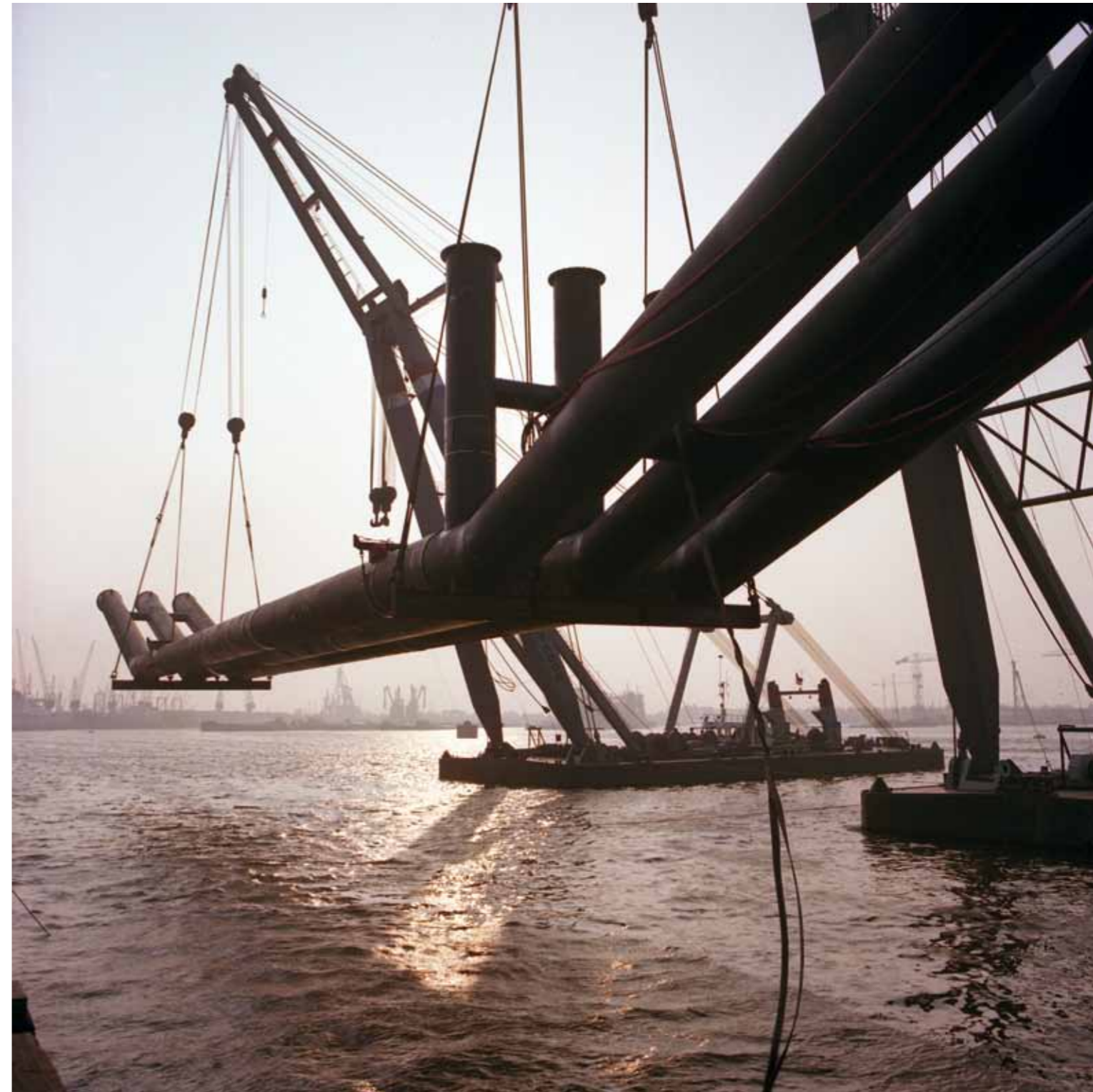
A new culvert for Rijkswaterstaat departs from the Waalhaven to be shipped to Limburg as one complete installation.
