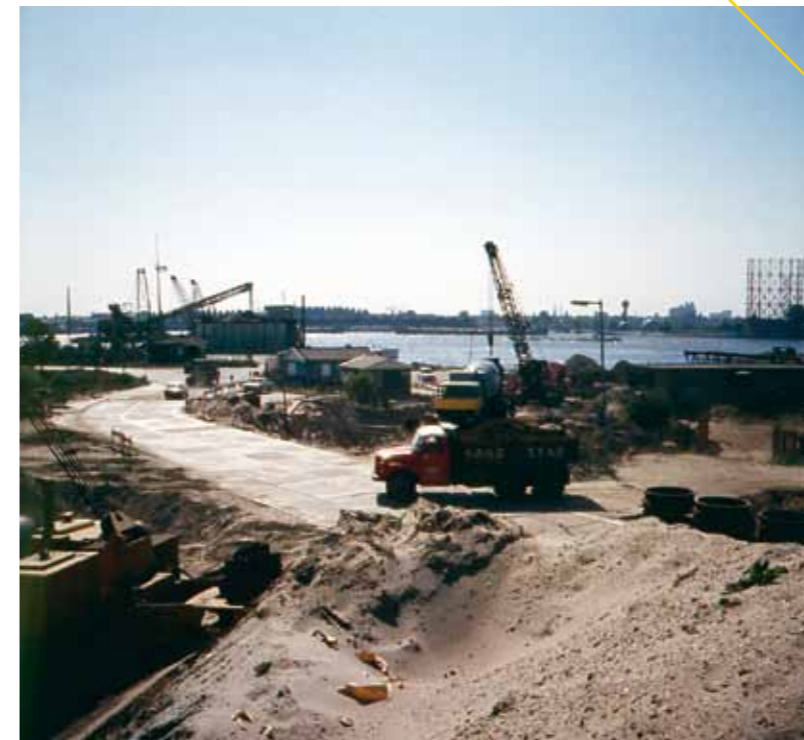
Construction of a double water pipeline at the Van Brienoord bridge in Rotterdam.
