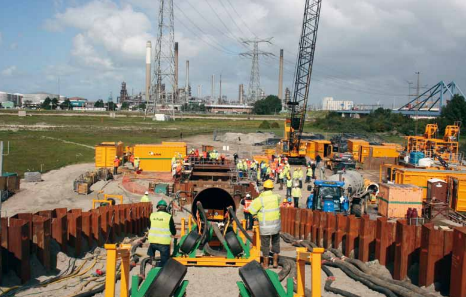
A.Hak Drillcon wins the NSTT No Dig Award with the direct pipe drilling under the Hartel Channel.
